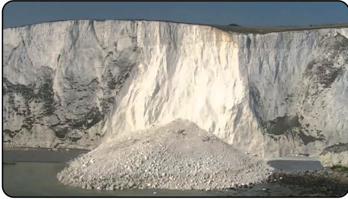
Figure 3 Rockfall at the White Cliffs of Dover
